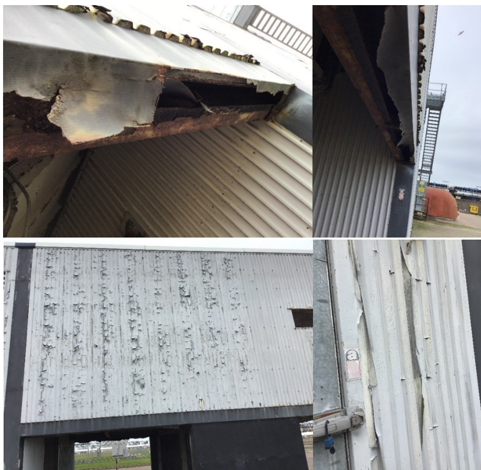
Figure 4: Coating breakdown of Galbestos cladding
